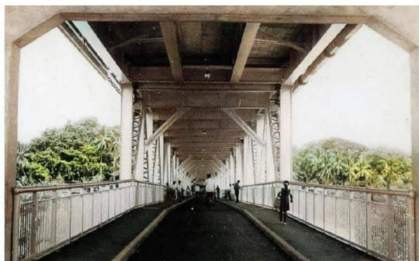
Many people use the lower deck of the old Kota Bridge to move between the northern and southern parts of Klang. (Klang Bandar DiRaja Facebook pic)
